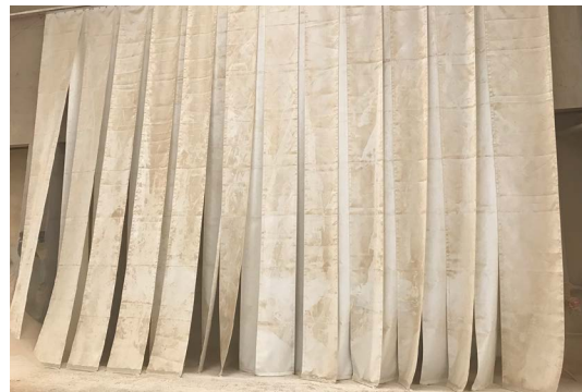
Dust curtains at Napier Works.
